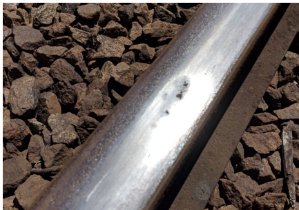
Fig. 1. Squat defect taken at Quorn, Leicestershire, UK railway station
